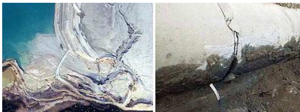
Figure 12: Aerial view of the embankment failure at Aitik (left) and the cracks in the decant conduit (right).
