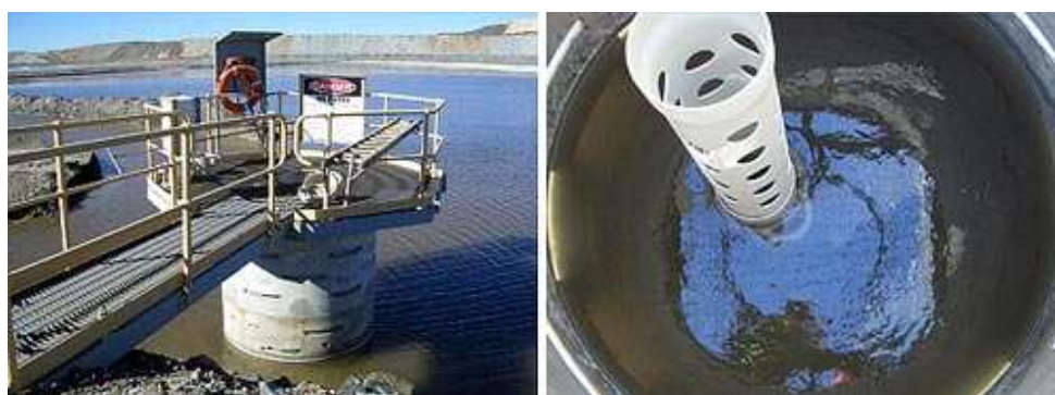
Figure 11: Decant tower with walkway (left), view inside the tower showing riser pipe and submerged decant collars (right).
