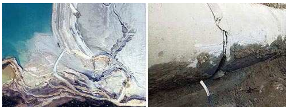
Figure 12: Aerial view of the embankment failure at Aitik (left) and the cracks in the decant conduit (right).
