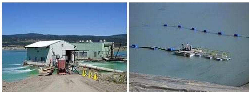
Figure 13: Fixed decant barge (left) and a mobile barge (right).
